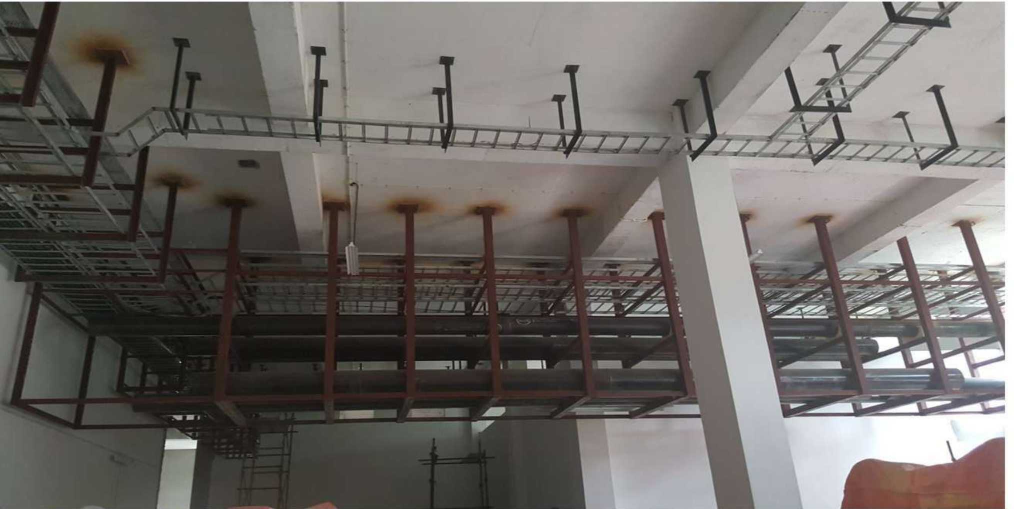
Two Tier Cable tray with structural Support
