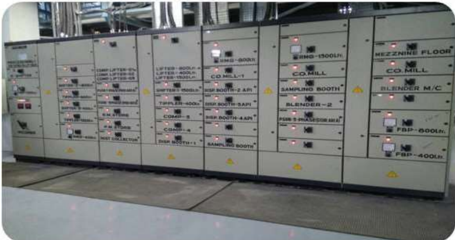
Low Voltage Panel Room
