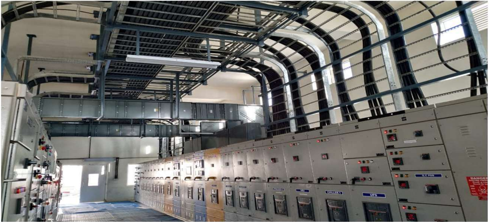
LT Panel Room with Top Cable Entry
