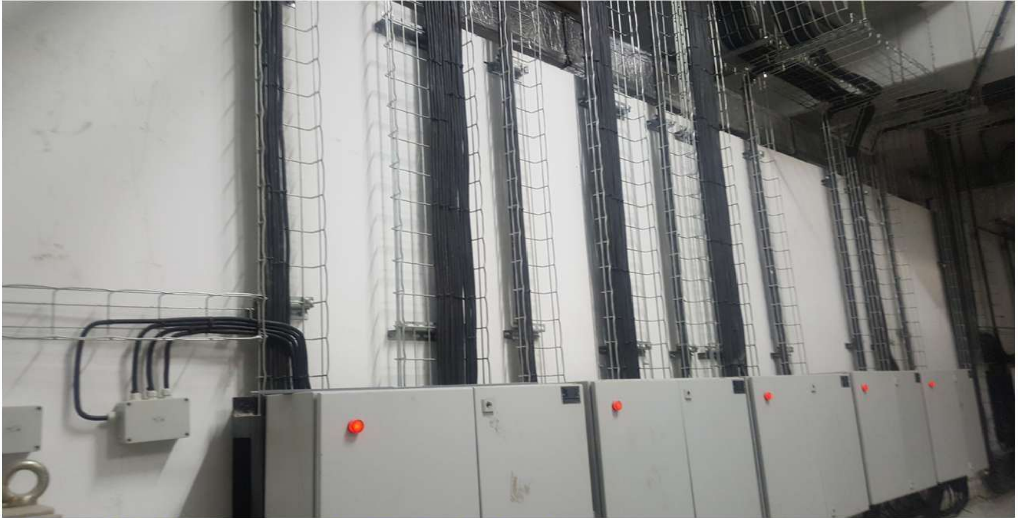
Wire mesh Cable tray connected to Distribution Boards
