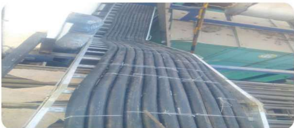
Cable Tray from Rack
