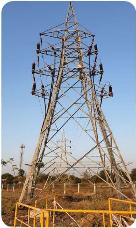
Lattice type 66kV Tower
