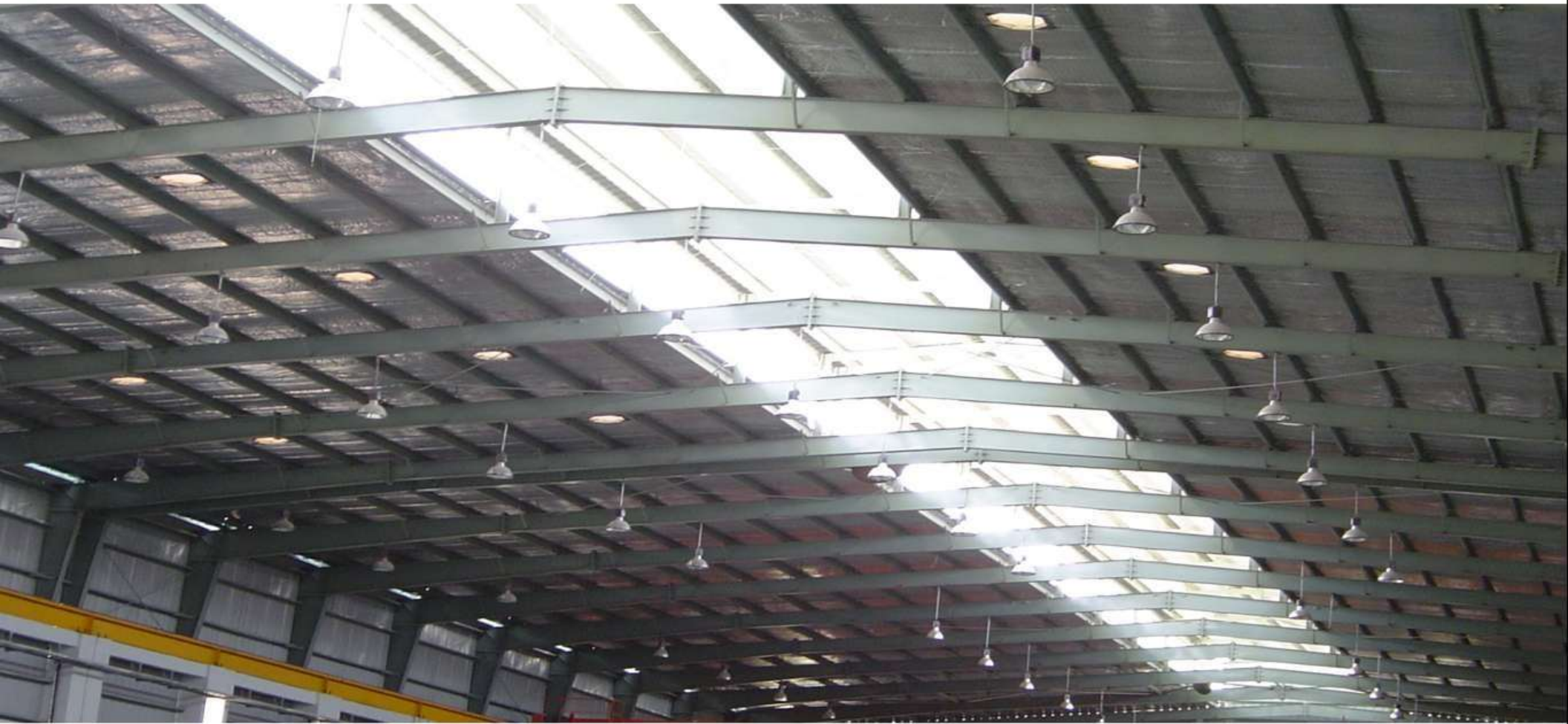
Ware House Lighting
