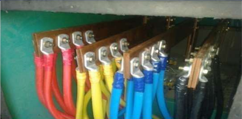
Low Voltage Cable Connections
