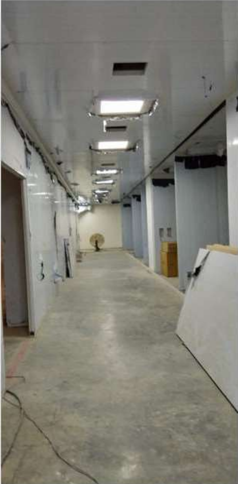
Clean Room Lighting
