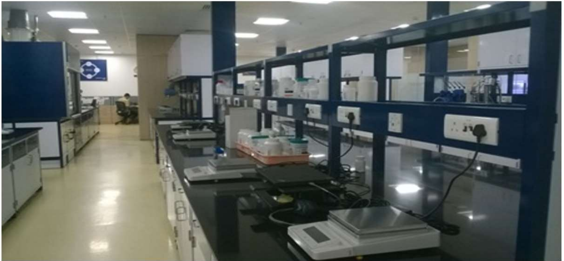
Laboratory Lighting & Power point Distribution
