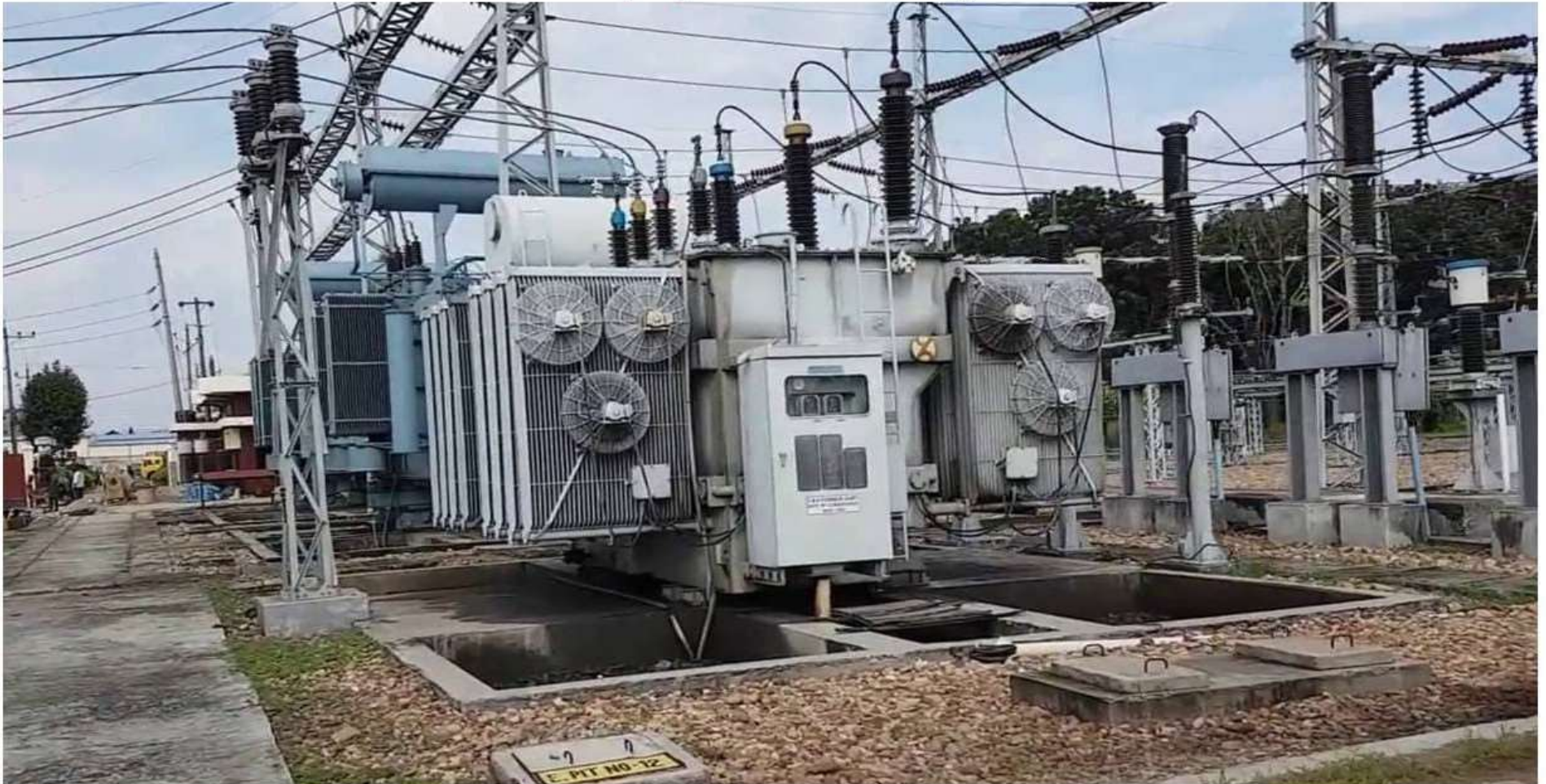
20MVA ,66 / 11kV Substation;
