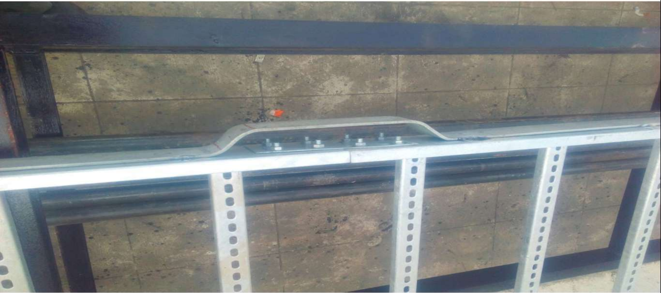
Cable Tray with Earthing Strip
