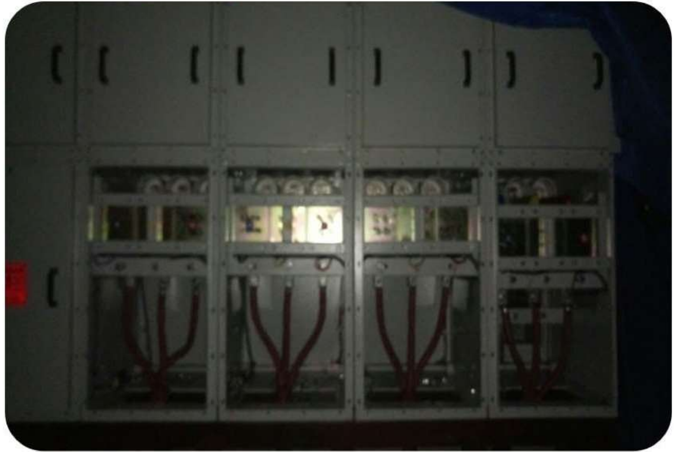
High Voltage Panel and Cable Termination
